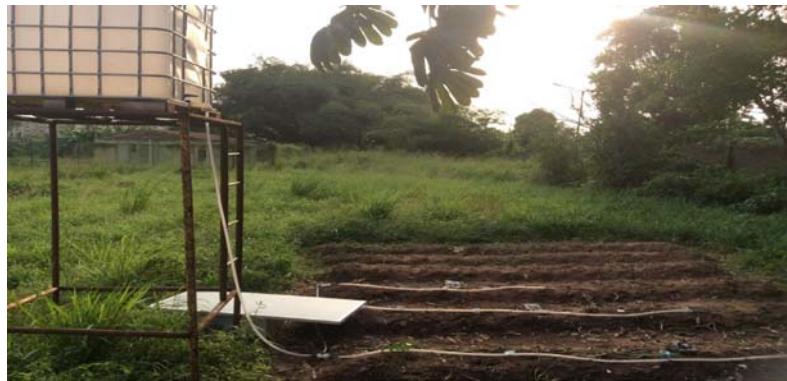
Figure 3.3: Automated irrigation system
